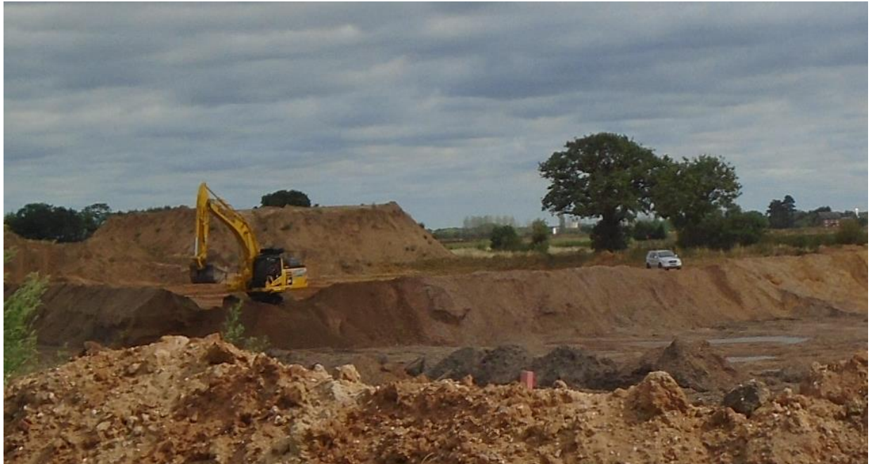
Figure 4: View of recent excavation of sand and gravel from land south of Roddige Lane
